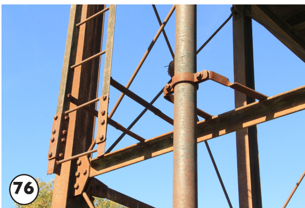
Method of fixing inlet pipe and ladder to the stand to bracing.
