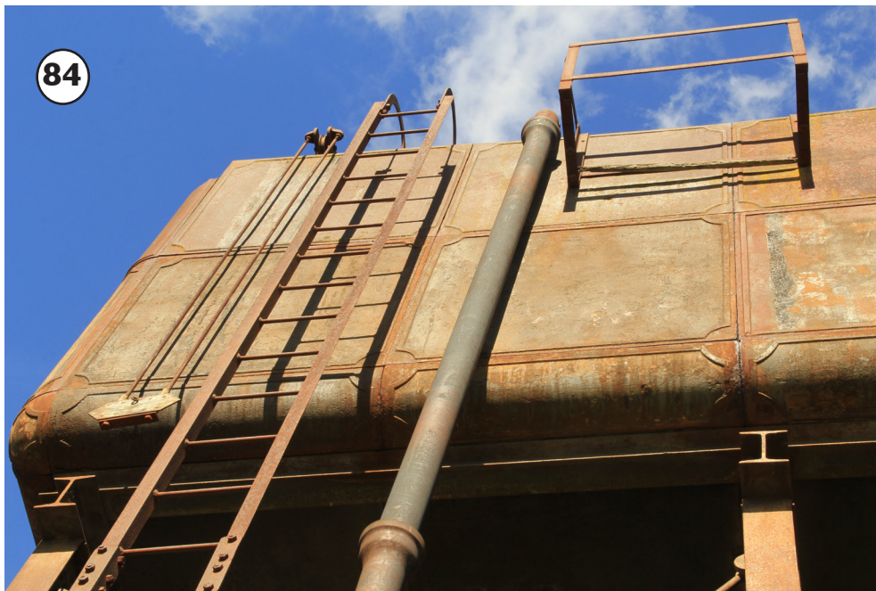
2-tier tank at Orange showing the 6" inlet pipe and indicator (note that this is a different style of pulley assembly)
